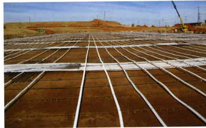
FIGURE 2.4-1 Post-Tensioned Slab Reinforced with Grouted Tendons, Ready to Receive Concrete (VSL; P141)
