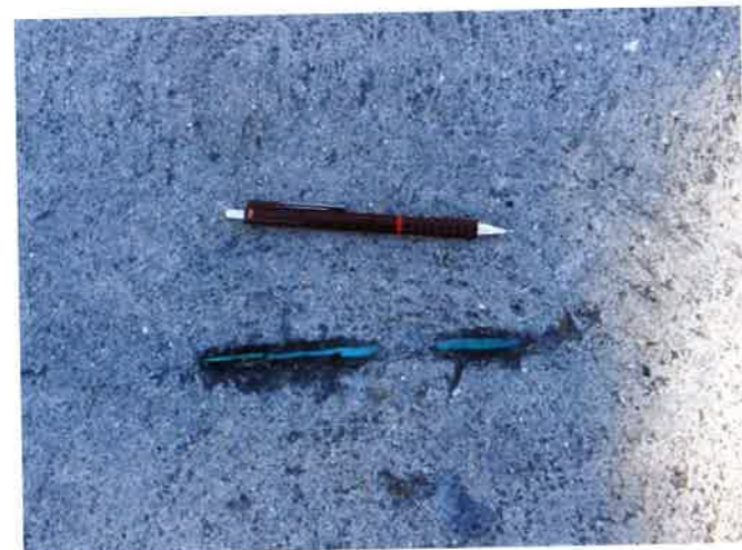
(a) Parking structure deck with exposed tendon (Palo Alto, CA; P264)
