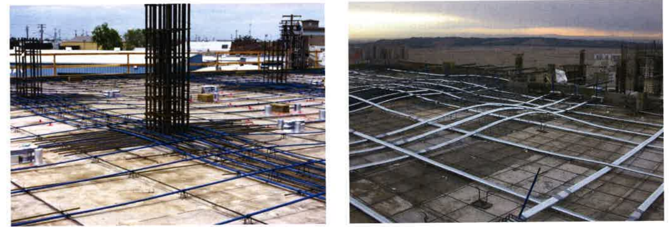
(a) Slab reinforced with unbonded tendons (b) Slab reinforced with grouted tendons (Tehran)
