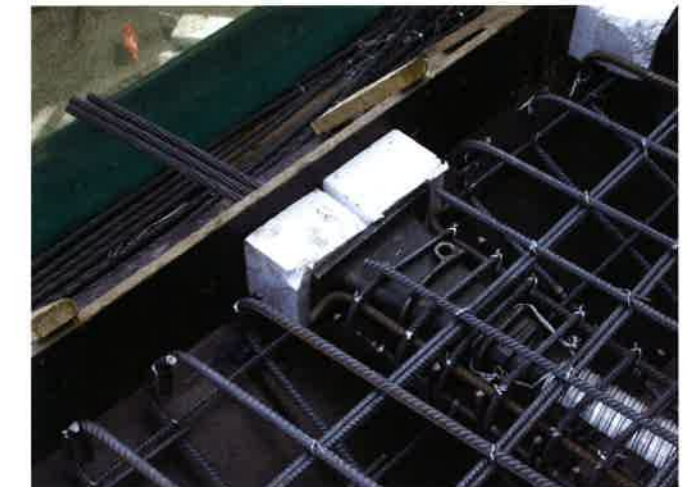
(a) Live end anchorage of a flat duct at slab edge (P146a)
