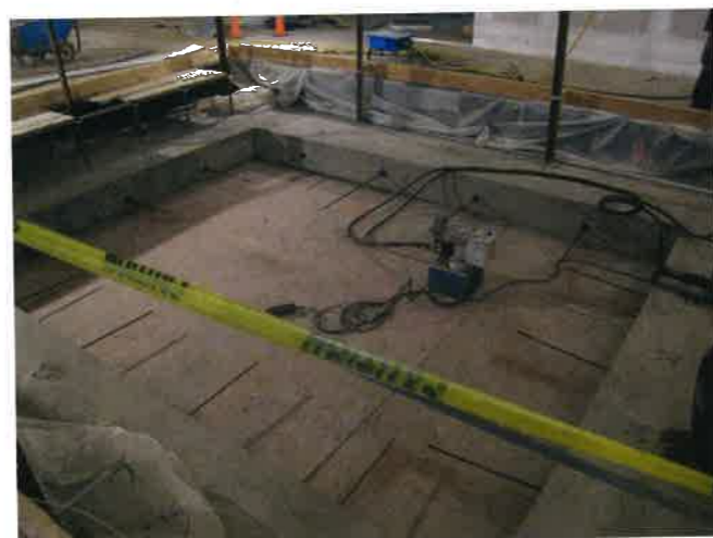
(b) View of opening showing anchored tendons (P479)
