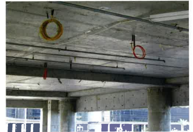
(b) Redundant beam between slab and downturned apron (Dubai; P319)
