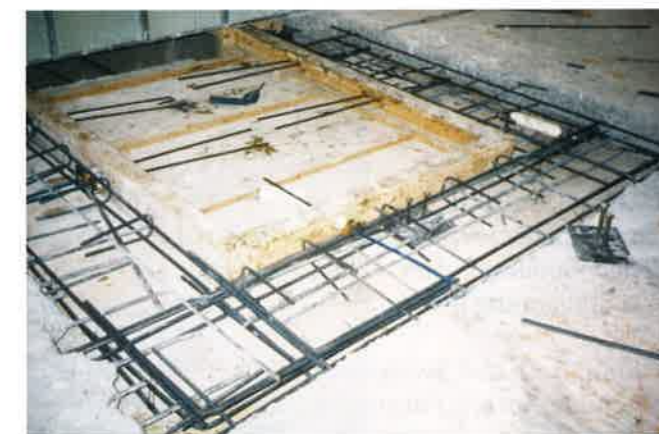
FIGURE 2.7.2-4 Tendons are De-stressed and Re-anchored at the Edge of an Opening (P481)
