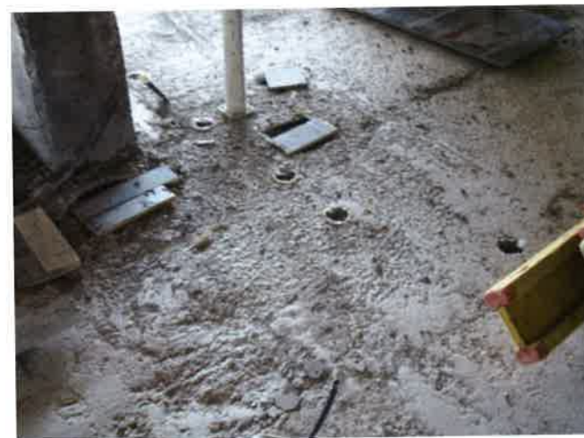
FIGURE 2.5.2E-2 Surface is Rough Finished in Anticipation of Mortar and Tile/Stone Topping (P193)
