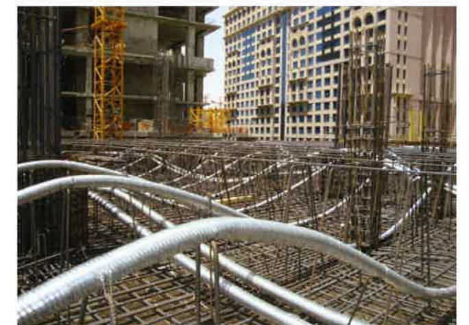
FIGURE 2.3.4-7 Construction View of a Transfer Plate 1.5 m (5 ft) Thick (Courtesy Freyssinet Gulf; ADAPT; Jabal Omar, KSA; P366)
