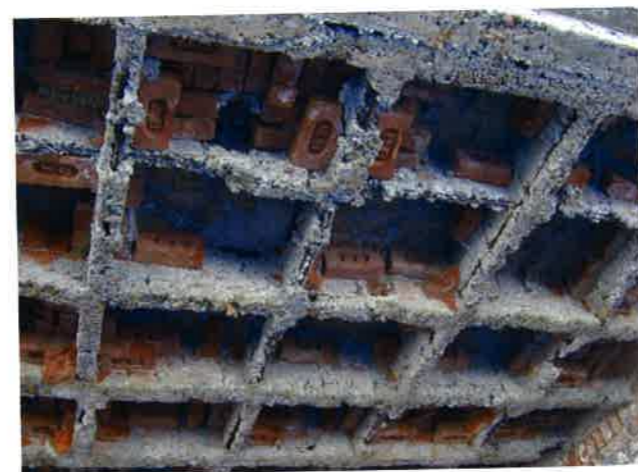
FIGURE 4.6.1A-2 Waffle Slab Construction in Himalayas (India; P276). Bricks on form provide the voids. Bricks that stick to cast concrete are left in place.
