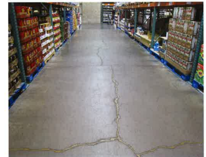
FIGURE 2.3.6-3 Example of Conventionally Reinforced Industrial Floor Slab with Extensive Cracking (P372)
