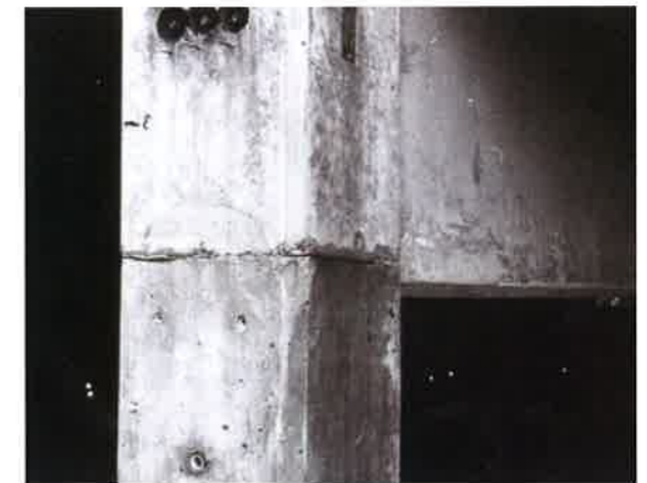
(a) Physical hinge at column-beam connection
