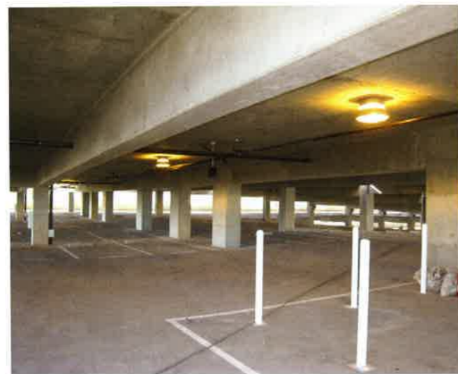
FIGURE 2.3.2-2 Interior View of a Beam and Slab Parking Structure (San Francisco Airport; P356)
