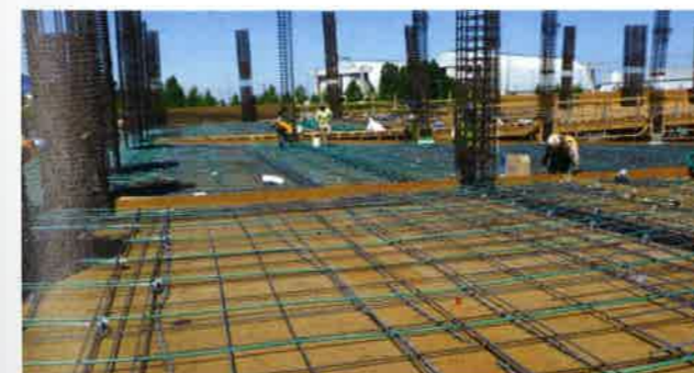
FIGURE 4.6.1B-2 View of a Typical One-Way Slab and Beam Construction for a Parking Structure in California. (beam are 65 ft (19.81m) long; 20 ft (6.10 m) apart; slab is 5.5" (140 mm) thick. Long plastic strips support the tendons at design height (P277)
