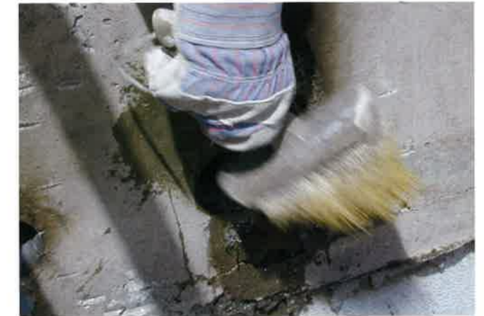
(b) Water is splashed into the recess block using a brush (P261)
