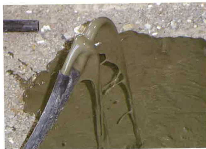
FIGURE 2.5.2K-3 Grout is Allowed to Spill Out of a Vent to Check its Consistency Prior to Locking it Off (P204e)
