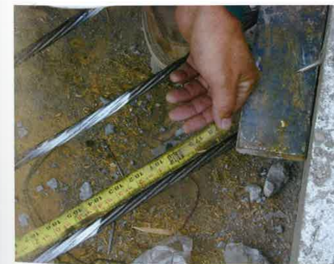
FIGURE 2.5.1J-2 Measurement of Elongation of a Strand that Exits the slab at an Angle (P445)
