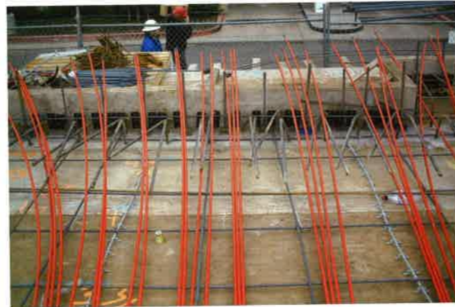
(b) Tendons are lined up with the anchorage devices, ready to be cut and threaded through (P421)
