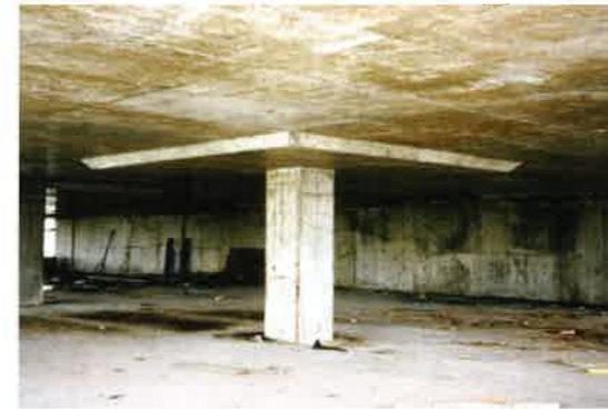
(c) View of a drop panel for improved negative moment capacity at support (P288)
