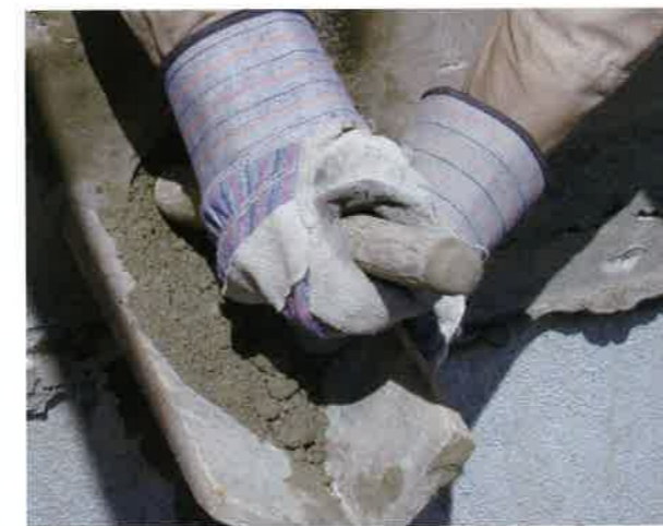
(c) Shrinkage compensating, stiff grout is pounded onto the recess block (P262)
