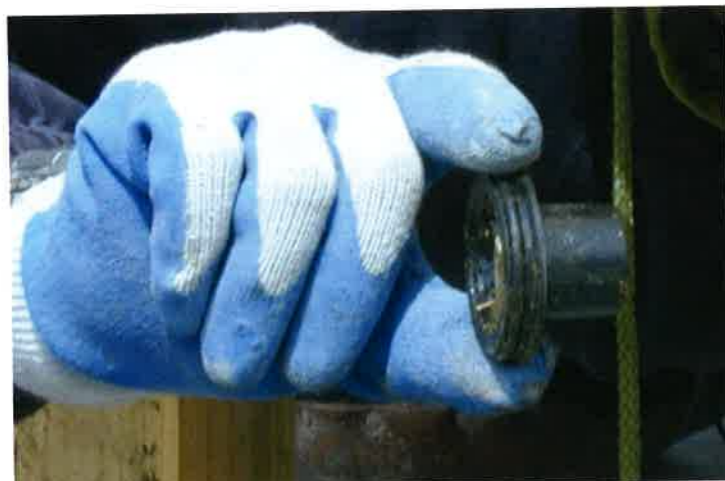
(c) A grease cap is used to cover the exposed metal (P458)
