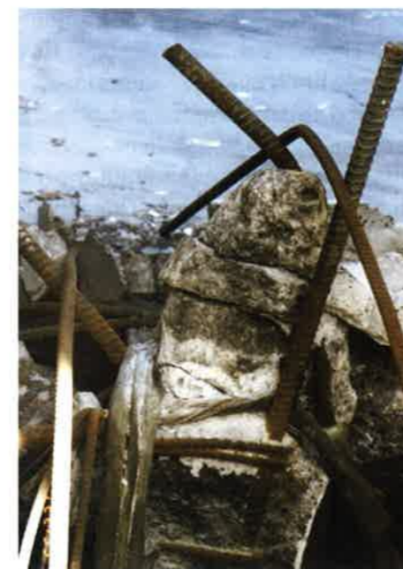
FIGURE 4.8.8B-1 Collapse of Slab Prevented by Tendons Passing Over the Column (Northridge Earthquake; CA; P335)
