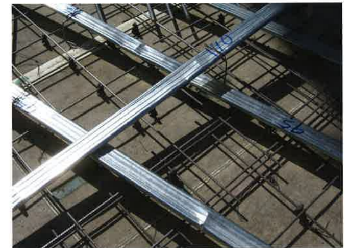
FIGURE 2.5.2D-2 Local Collapse of Duct from Rough Handling (P476)
