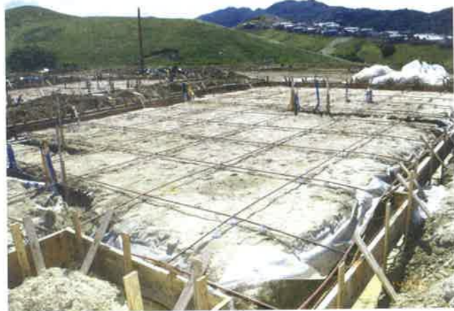
FIGURE 2.3.7-6 Example of a Post-Tensioned SOG Ready to be Cast, California (Common dimensions are 7 to 8 in (180 to 200 mm) for the uniform slab thickness with perimeter beams 12 in (300 mm) deep and 10 in (250 mm) wide; P378a)
