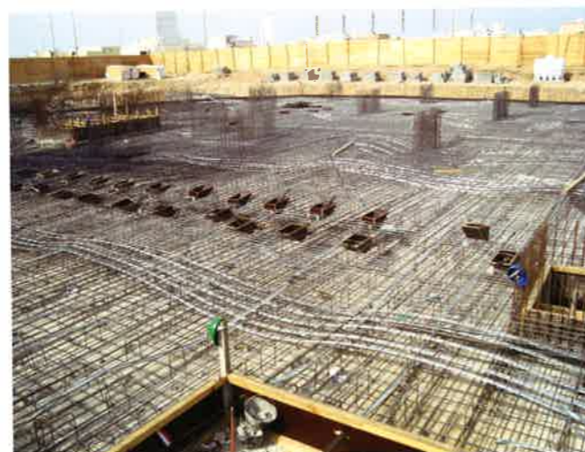
FIGURE 2.3.5-4 Example of a Mat Foundation in KSA Using Grouted Tendons (Freyssinet Gulf; P369)
