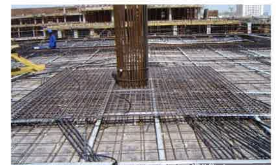
FIGURE 4.8.8B-4 Congested Column Cage Prevents Passage of Tendon over Column (P338)
