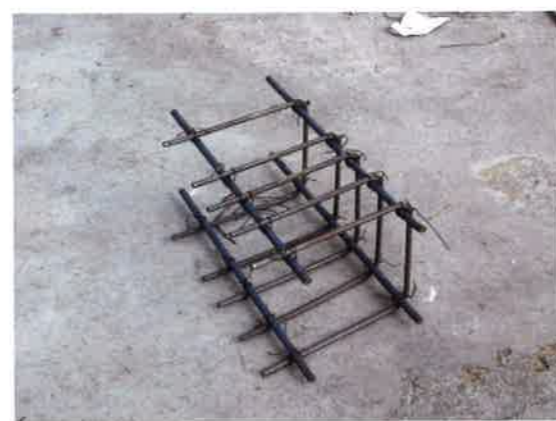
(d) View of a pre-assembled cage for bursting reinforcement of grouped unbonded tendons (P595)
