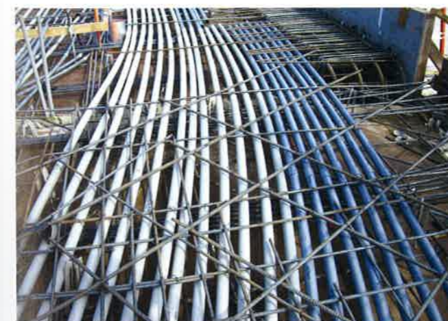
FIGURE 2.5.1D-3 Crowded Placement of Electrical and Data Conduits in a Thin Slab (P427)
