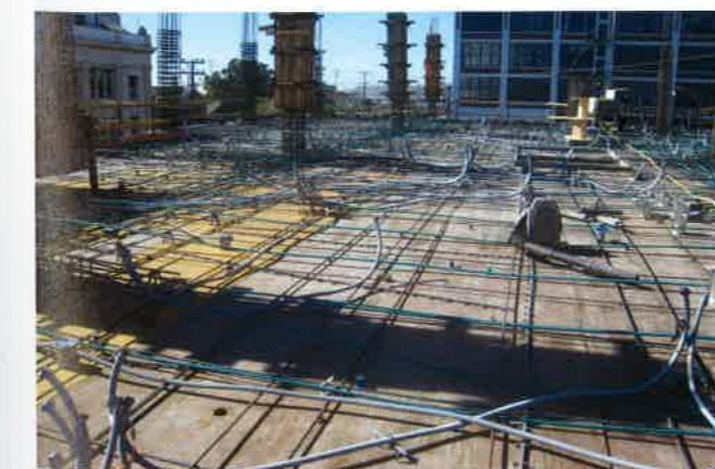
FIGURE 2.6.2B-1 Slab ready to Receive Concrete (Courtesy Nishkian Menninger; Portero; San Francisco; P213)
