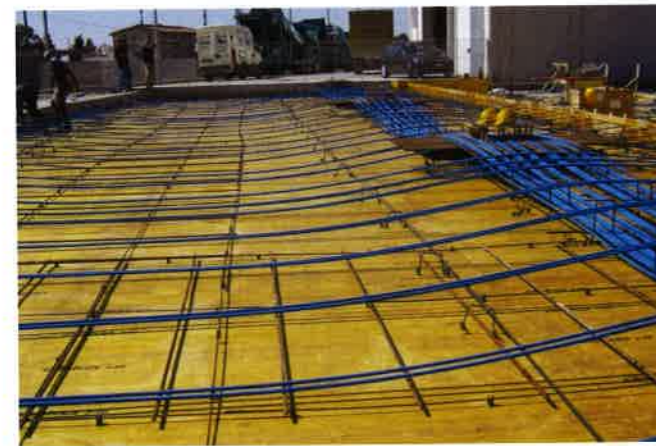
FIGURE 2.4-2 Post-Tensioned Slab, Reinforced with Unbonded Tendons, Ready to Receive Concrete (Courtesy of GRANDI STRUCTURE S.r.l. Italy; P142)
