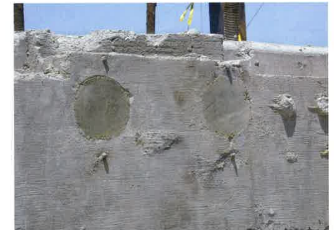
(d) The recess is finished off with a smooth surface in line with concrete slab (P263)
