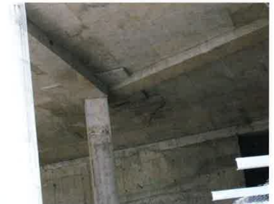
FIGURE 4.6.3-3 Example of a Non-effective Column Drop to Enhance Punching Shear Capacity (Trump Tower, Panama; P510)
