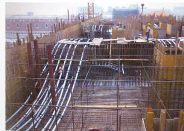
FIGURE 2.3.4-5 Transfer Plate Showing Both the 1 m Bottom Layer Tendons and the Full Height Tendons (P364)
