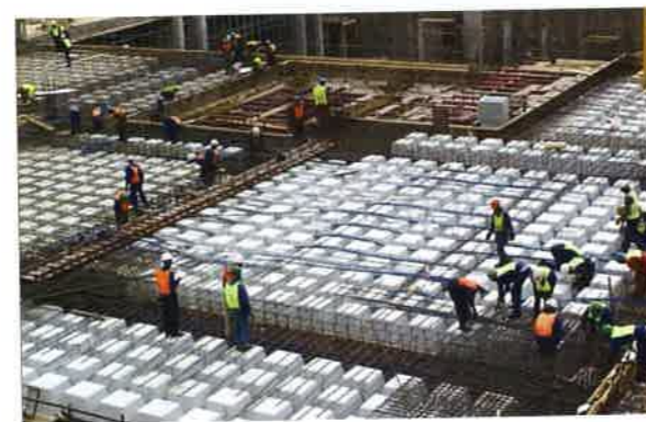
(b) Construction of a post-tensioned waffle slab (South Africa; Vstructural; Courtesy Graemer; P291)
