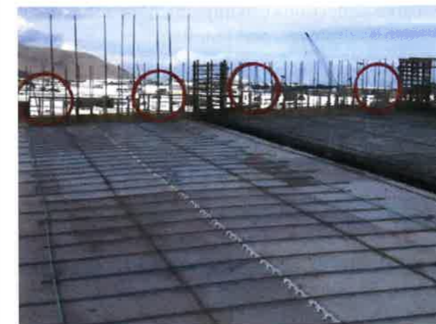
FIGURE 4.10.5.3B-2 Construction of a One-Way System, where Bars are More Uniformly Spaced (P244)
