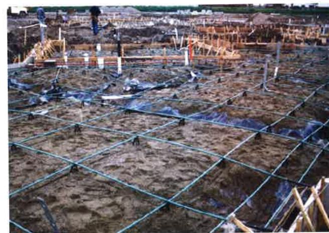
FIGURE 2.3.7-7 Example of a Post-Tensioned SOG Foundation in Texas. (Slab 4 to 5 in thick (100 to 130 mm), beams 12 to 15 ft (3.6 to 4.5 m) apart tendons 4 to 5 ft spacing (1,200 to 1,500 mm)) (P379)
