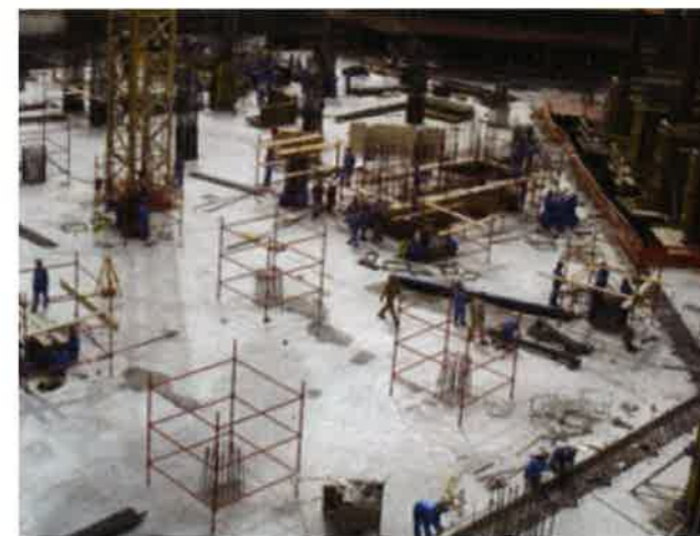
(b) Podium provided with closure strip to control cracking (P313b)
