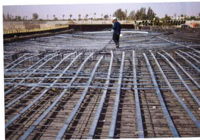
FIGURE 2.5.2-4 Tendon Layout of a Heavily Loaded Slab Using Grouted Tendons The close spacing of the tendons in the distributed direction reflects the heavy design load of slab (Courtesy Freyssinet Gulf; P693)
