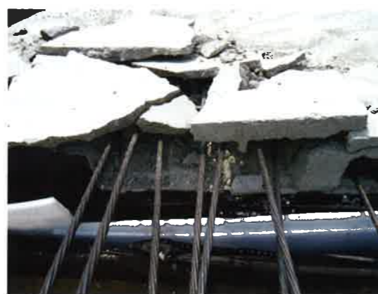
(b) Bursting of slab behind grouped tendons (South Korea P673)
