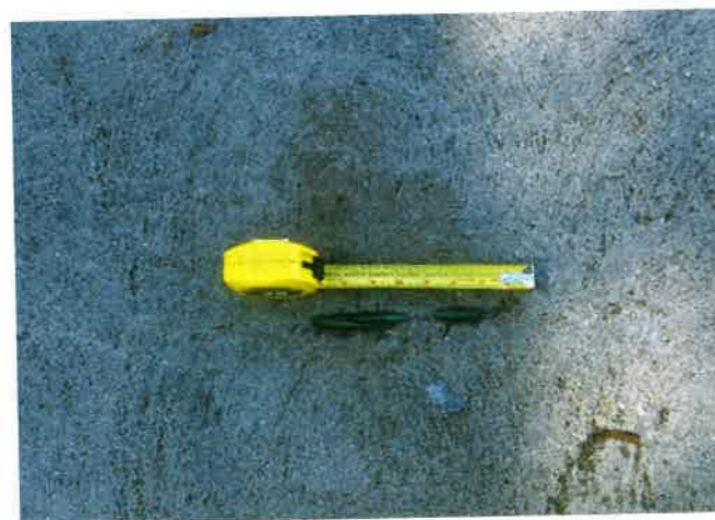
(b) Exposed tendon on parking deck (San Jose, CA; P706a)
