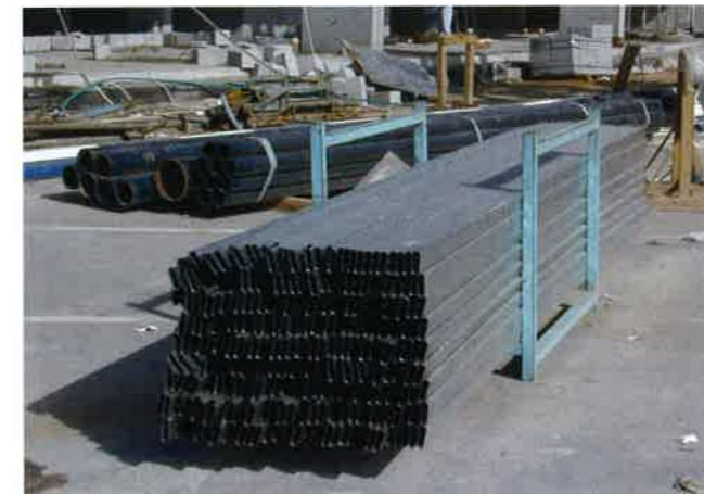
FIGURE 2.5.2A-1 Bundle of Flat Ducts Delivered to Site (P168)
