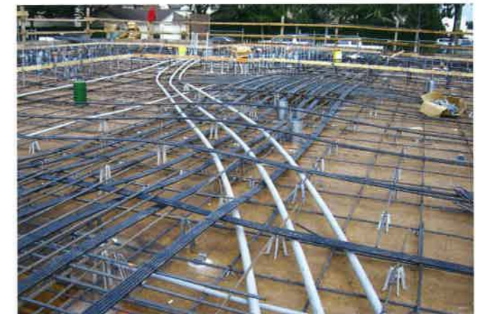
FIGURE 2.5.1D-2 Electrical and Data Conduits in Slab (P426)
