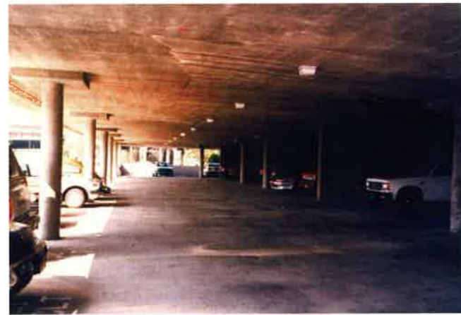
(b) Level below the steel frame superstructure featuring support arrangement for parking (P137b)
