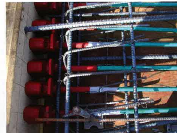
FIGURE 4.4.1.3-2 Example of Application of a post-tensioning System in Use in a "Corrosive" Environment (P502)
