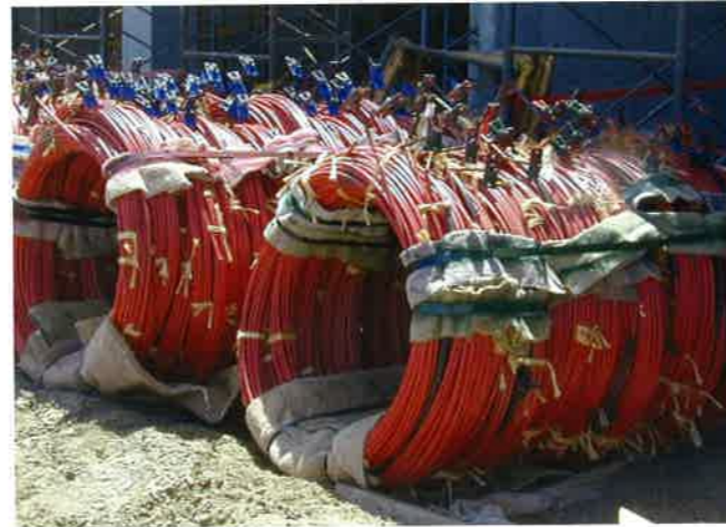
FIGURE 2.5.1A-1 Tendons are Cut to Size; Provided with Dead End Anchor; Grouped; Tagged, and Delivered to Job Site (P402)
