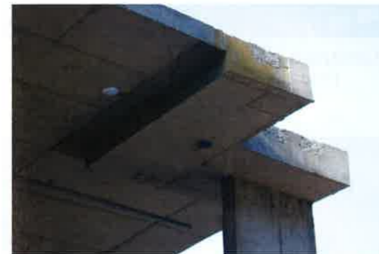
(d) Strengthening around a non-standard column support configuration for improved shear transfer (P509)
