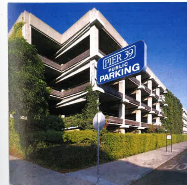
FIGURE 2.3.8A-2 Pier 39 Parking Structure Blocks at the outer face of the columns are anchorages of the externally applied tendons (San Francisco, California; P381)
