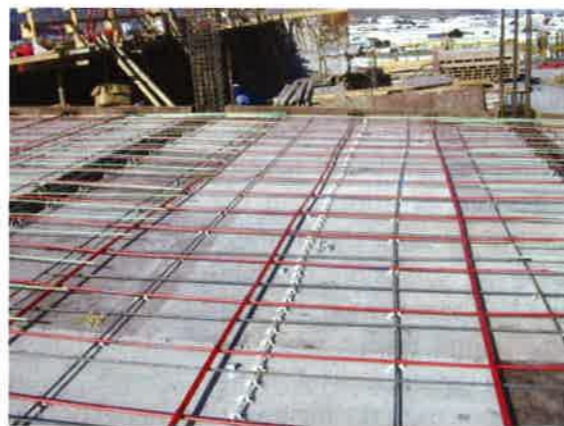
FIGURE 4.8.4-4 Disadvantageous Slab Tendons between Post-Tensioned Beams (P326)
