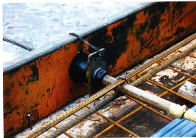
(c) Live end, corrosive (P153c)
