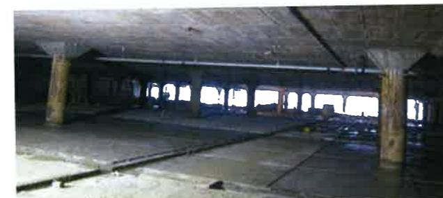
(b) View of a tapered column drop used for punching shear (Kolkata) (P287)
