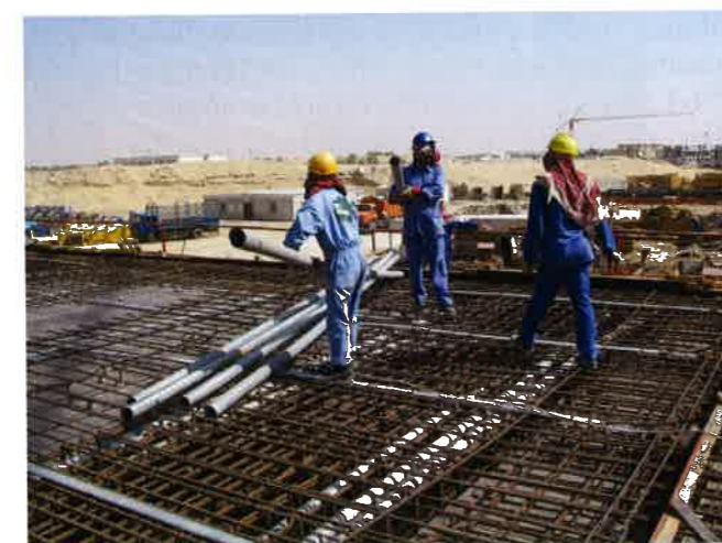
FIGURE 2.4-3 Multi-Strand Construction for a Department Store, Dubai (Courtesy of Freyssinet Gulf; P143)
