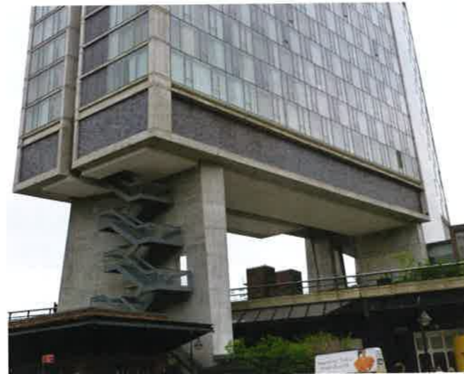
FIGURE 2.3.4-2 View of a Transfer Plate that Straddles a Viaduct (New York; P492)
