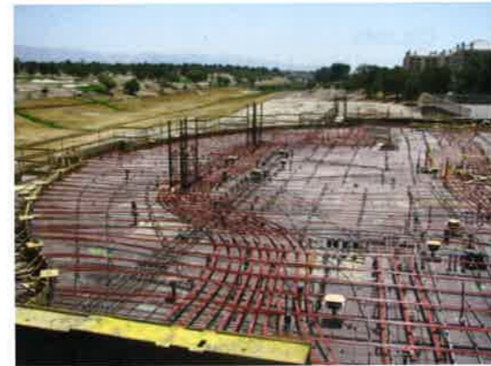
FIGURE 4.8.8A-7 Grouping of Tendons in Direction, where Supports do not Line Up (Indian Well, USA; P334)
