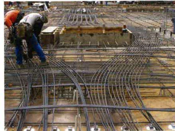
FIGURE 4.8.9F-5 Swerving of Unbonded Tendons to bypass an obstruction (Valencia Building, San Jose, CA; P232)
