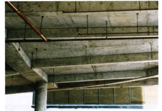
(a) Superfluous beam framing for a post-tensioned parking structure floor (P666)
