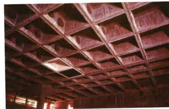
(a) Construction of a post-tensioned waffle slab (Moscone Center San Francisco; P290)
