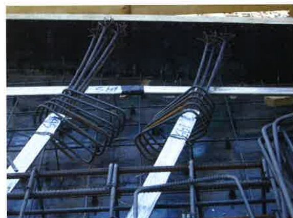
(a) Bursting steel being arranged behind dead end of a grouted flat duct tendon (P593)
