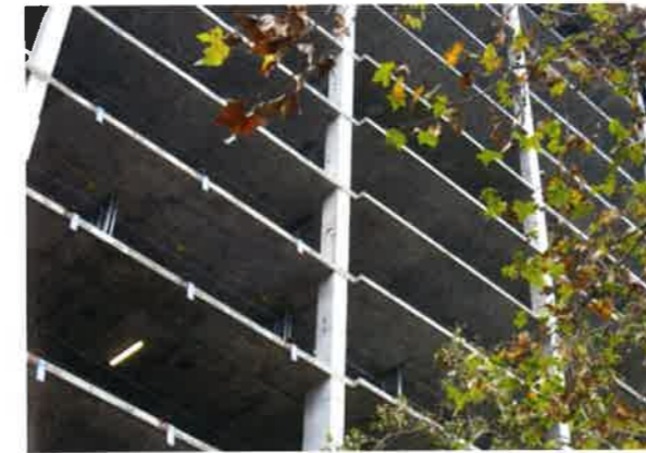
FIGURE 4.6.6A-4 View of a Beamless Floor System in a High Seismic Risk Region. Shear Walls Provide the Lateral Force Resisting System (San Francisco Bay Area; P306)
