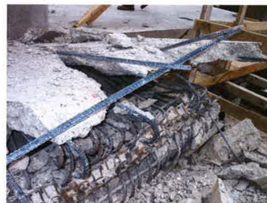
(a) Bursting of slab behind grouped tendons (US, P672)
