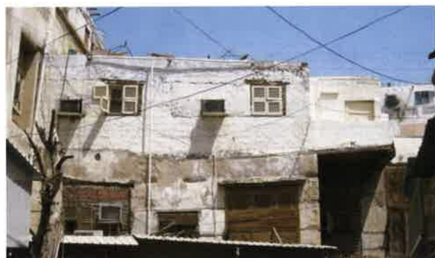
FIGURE 4.10.6.3A-1 Noticeable Out-of-Level Displacement of a Floor (KSA; P249)
