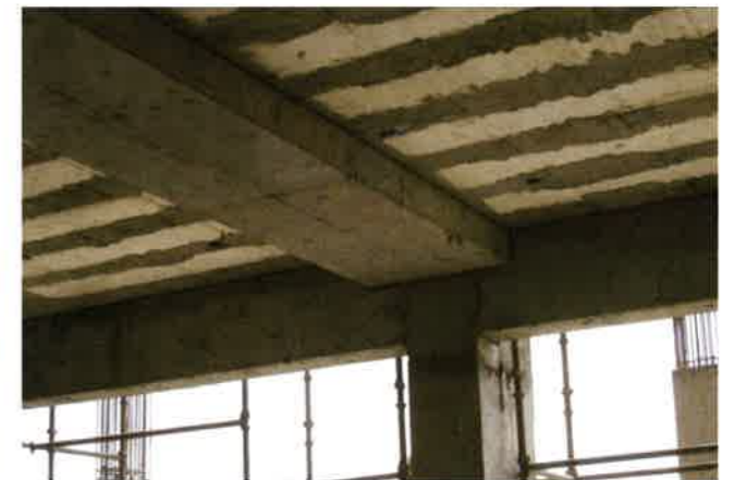
FIGURE 4.6.1B-5 Example of a Post-tensioned Floor System with Slab Band and Void Creating Foams (P281)
