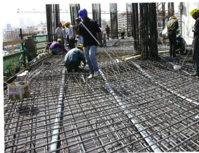
FIGURE 2.6.1A-1 View of Reinforcement in a Floor System Ready to Receive Concrete (Beirut; P208)
