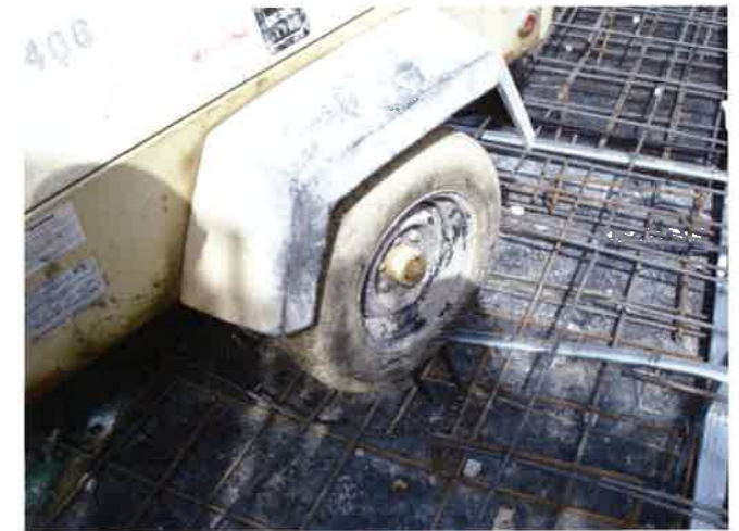
FIGURE 2.5.2D-1 Rough Handling of Ducts in Place Results in Duct Collapse and Damage (P475a)
